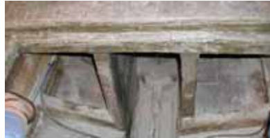
ARG installation surface (side view)
