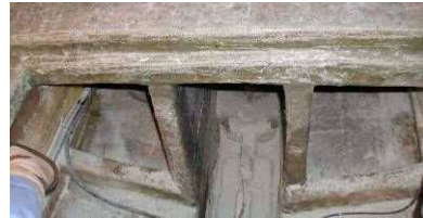
ARG installation surface (side view)
