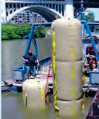
Custom Vertical Pontoons manufactured to allow accurate horizontal control during large pipe and valve maintenance and assembly
