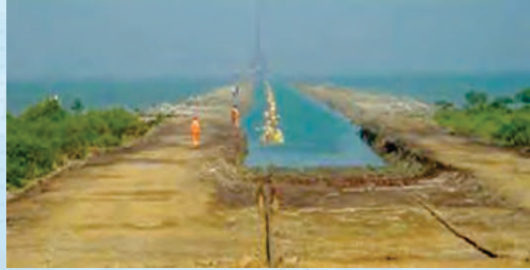
Installation of oil pipeline in the Middle East using Salvage Pontoons 6,000 lbs.
