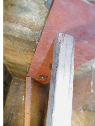
ARG installation surface (bottom view)
